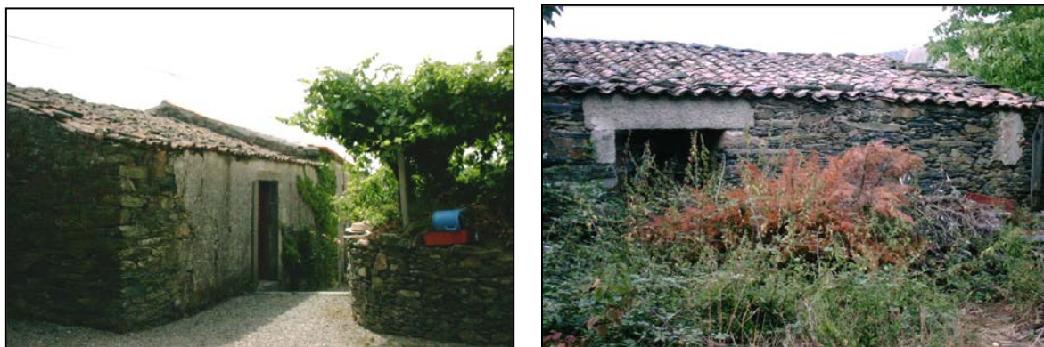
Fig. 4 - The situation before the project (photos by Jerónimo Pimentel and Manuel Villas-Boas).
