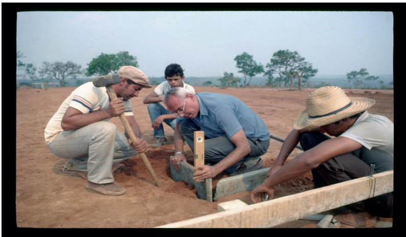
Abadiana experimental school system: Lele teaching the workers how to prepare the ground for putting up a column
