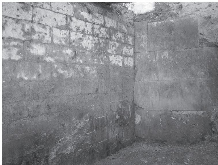
Fig. 6. Excavations at the Marstall bastion. Outer wall of the bastion flank with dolomite cladding. Excavation site in November 2015.
